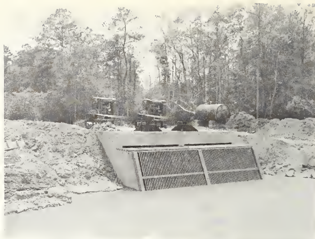
Low head drainage pumps and reinforced concrete pump structure and trash racks.
